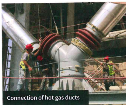
Hot gas outlet behind preheater
